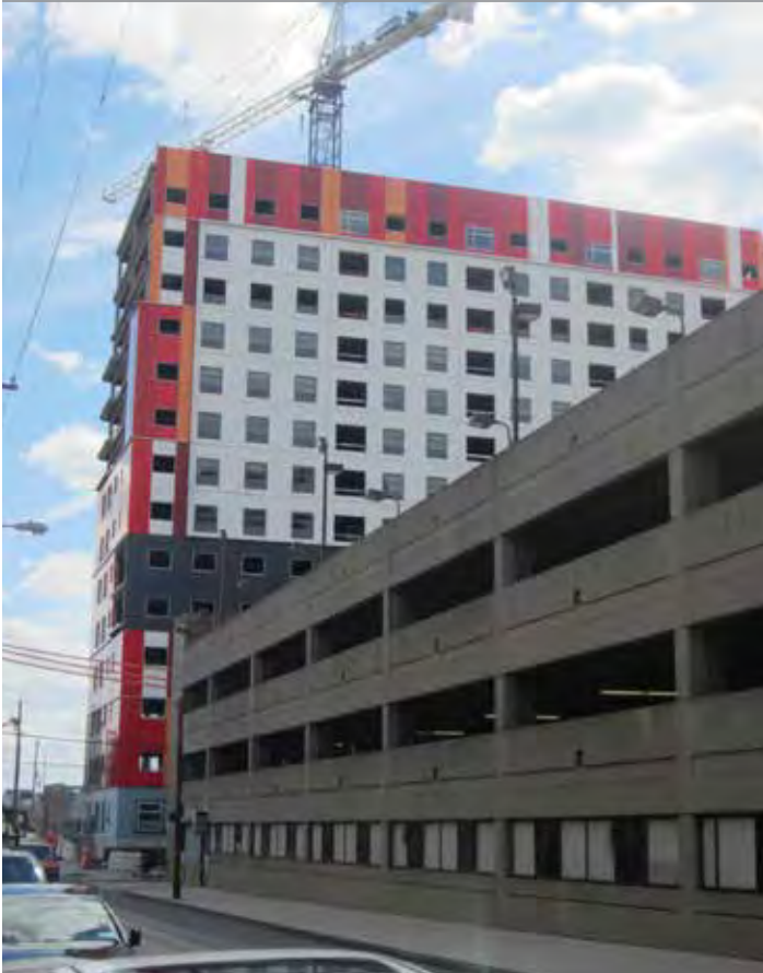
The 4.5-acre former Wanamaker Middle School site at 11th Street and Cecil B. Moore Avenue is being redeveloped into a mixed-use, privately owned student housing development for 2,500 students.
