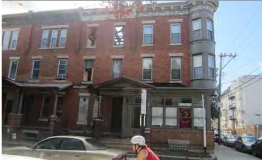
Even on well-maintained blocks such as Park Street, vacant, crumbling buildings detract from the overall character of the neighborhood, depress surrounding home values and hindering investment.
